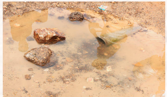
Leaking pipes force residents to collect water from unsafe sources. | Photo: Bekithemba Mpfu/The Citizen
